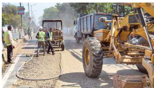
Workers carrying out road repair ahead of U.S. President Donald Trump's visit, in Agra on Monday. •PTI
